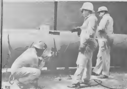
Welder M. Roga (left) and Boilermakers B. Kally (c) and C. Barnabela do their share of the work.
